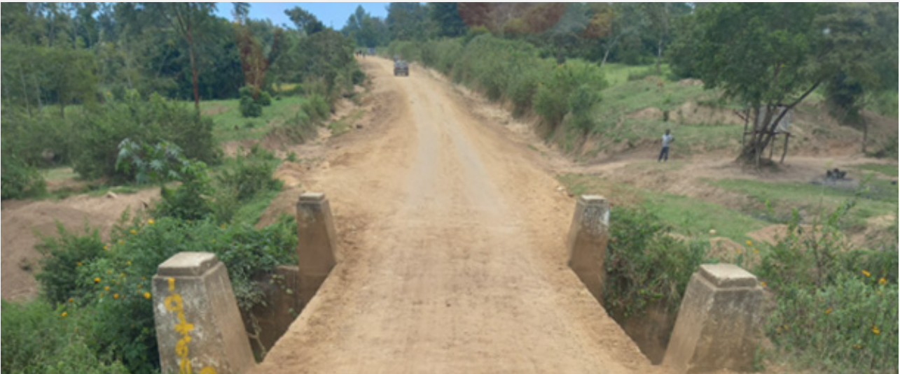
Single-lane bridge at Karisandeti along the Kimaeti – Lwakhakha road, there is a need to construct two-lane bridges along this road with capacity suitable for use by heavy commercial vehicles.
