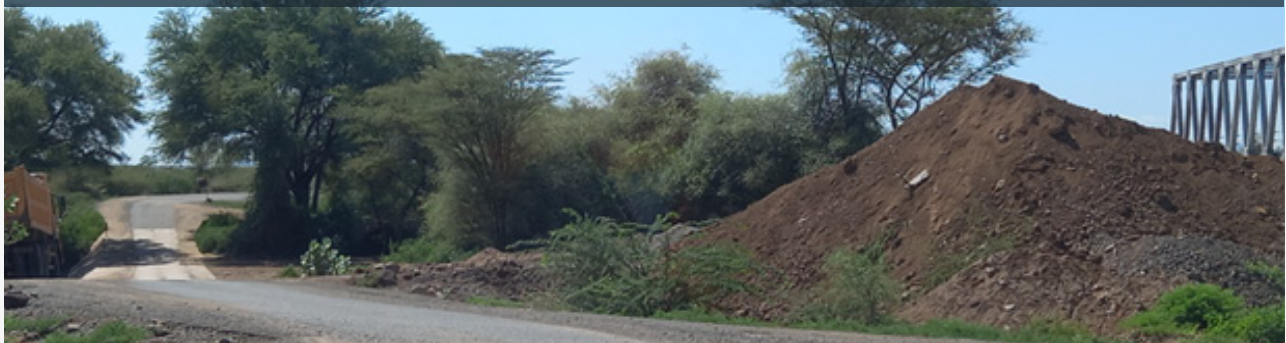
Below: On the left shows an existing road passing across a seasonal river; on the right, a truss bridge part of the new road is being constructed across the river.
