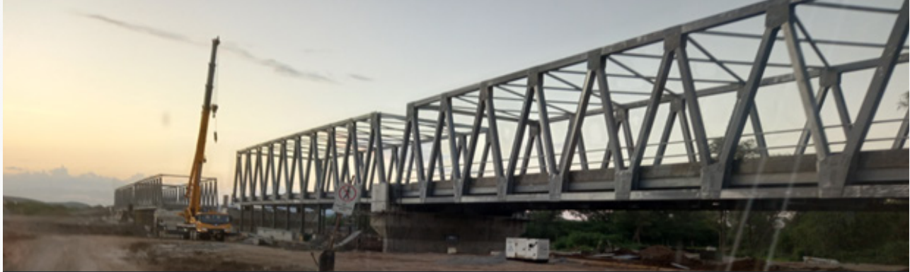
Above: A truss bridge under construction, abnormal loads of abnormal heights may not pass through this type of bridge.
