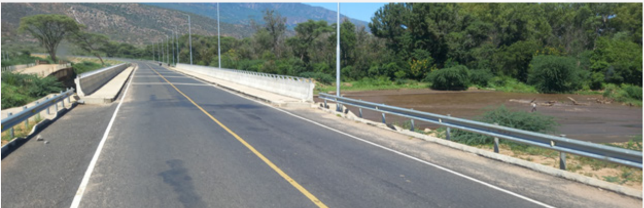
Heavy-duty bridge has been constructed at Kainuk, the river used to overflow the bridge that was previously there. The area experiences unpredictable flash floods. The new bridge gives peace of mind to users of this road; worries of finding the bridge awash have been addressed.
