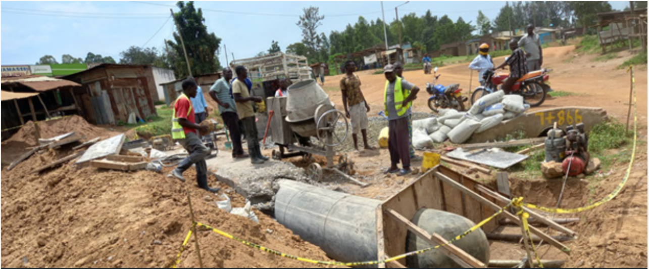
Culverts being constructed at Sango near Malakisi along a section of the alternative transit route from Kimaeti to Lwakhakha.
