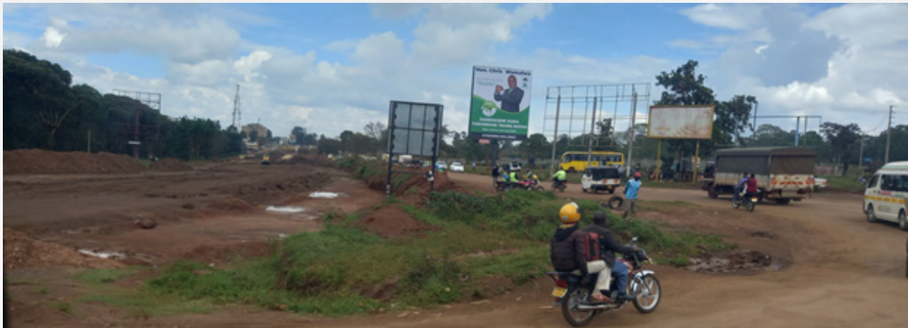
Part of the Kitale – Suam River road under construction. The distance from Kitale to the Suam River border station with Uganda is about 45Km, and the distance from Suam River Border station to Kapchorwa - Uganda is about 80Km.
