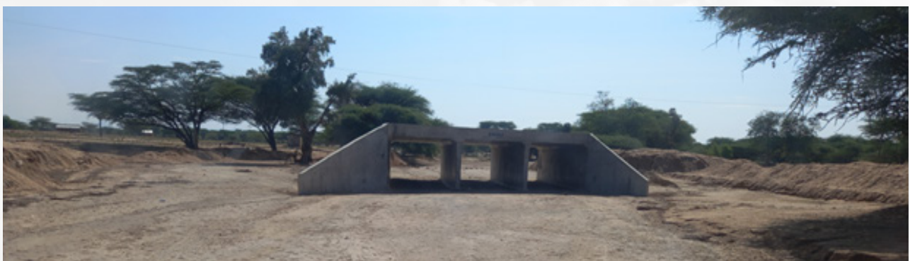
Bridge/Culvert does not cover the entire width of the seasonal river; what are the contractor's intentions?
