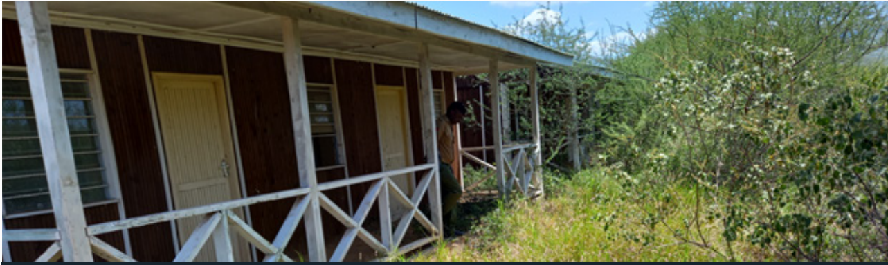
One of the staff houses, the houses are temporary structures in a poor state. How safe are staff in wooden houses where neighbouring local communities fight with live ammunition?
