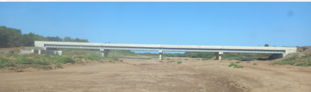
Several bridges are under construction between Lokichar and Nadapal as part of the Kitale – Nadapal road upgrade project.
