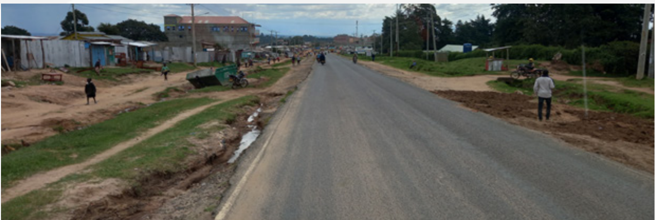
The Eldoret – Kitale road lacks shoulders, and along some sections, the road is being eaten away. As a result, cyclists are in danger of using this road. With gulleys on the side of the road, it is difficult to veer off the road to avoid a head-on collision.
