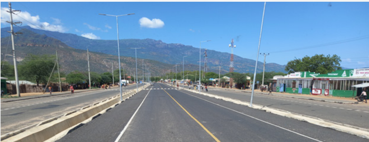
Dualling of road through Kainuk trading centre with main carriageway and service roads for vehicles that may wish to make a stop.
