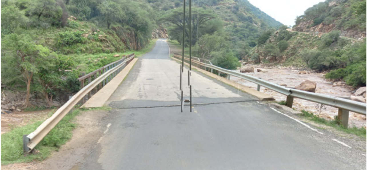
Some crash barriers were found not appropriate for the purpose they ought to serve.
