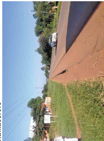
The very straight section prompts motorists to overspeed and overtake dangerously
