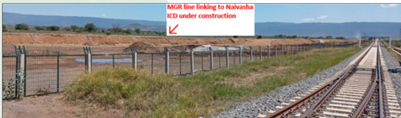
Above: Left MGR line connecting to Naivasha ICD under construction, Right is the SGR line entrance to Naivasha ICD
