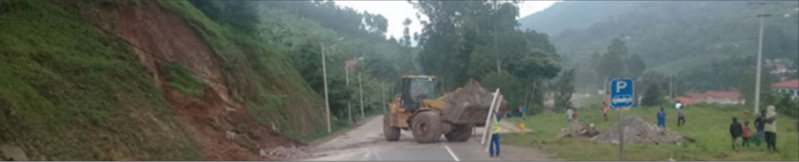
Above: A grader clearing the road after a landslide along the Kigali – Rubavu road. The Survey Team also encountered several landslides along the Kayonza-Bujumbura road after Kayonza town towards Bujumbura. With heavy rains due to the topography of the area several landslides occur which affect flow of traffic along these transit sections.
