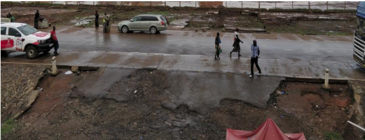
The Elegu- Nimule road being eaten away especially at places where feeder roads join it. Furthermore heavy trucks park along the road while awaiting clearance by customs to the detriment of the newly constructed road this is despite availability of ample parking space in the parking yards available at the border station.
