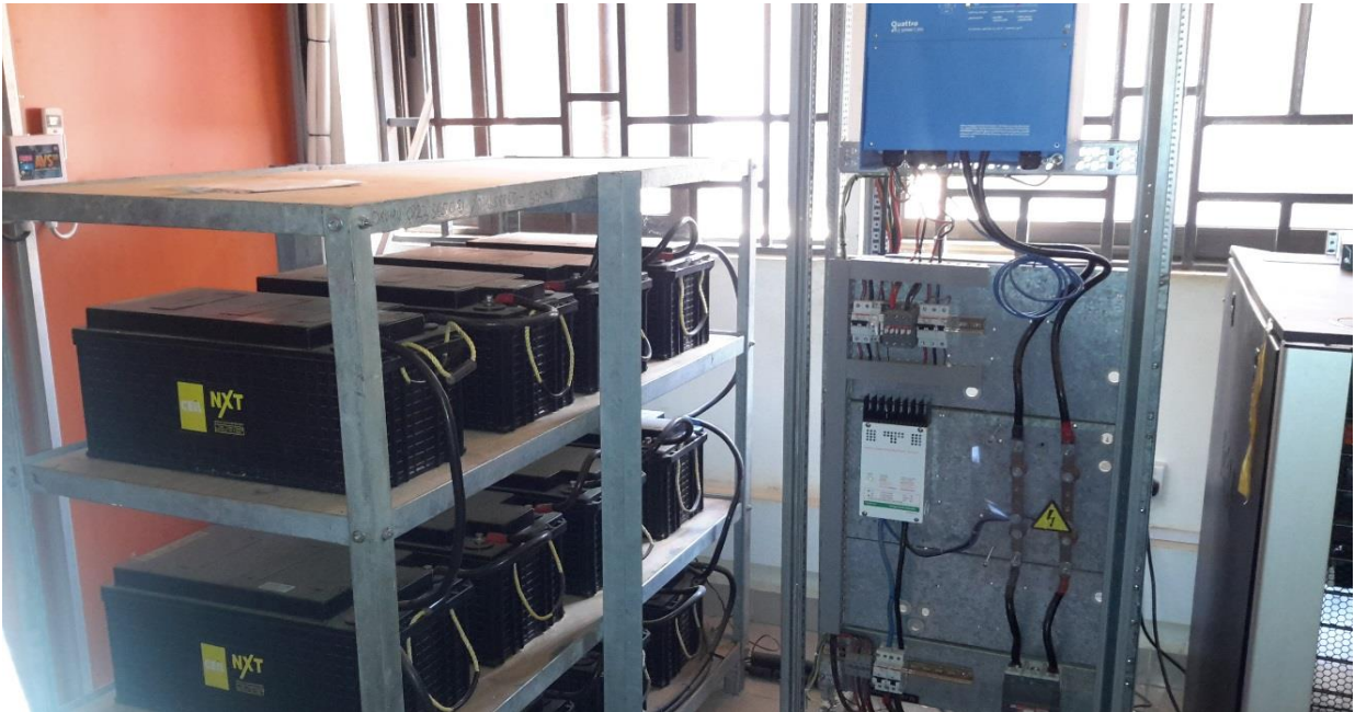
Solar power at Malaba OSBP: Promoting Green Environment by use of renewable energy
