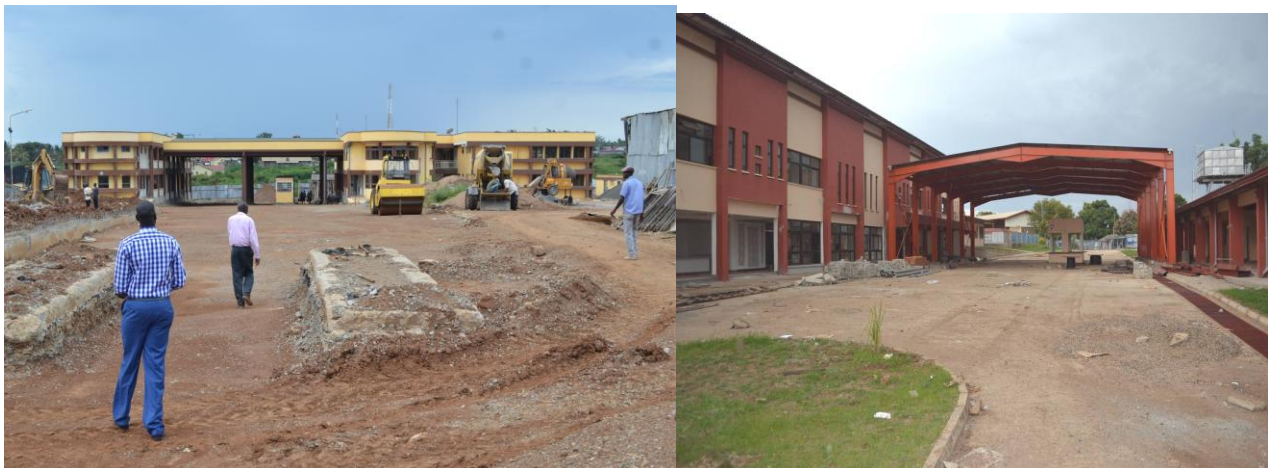
Above left , Malaba - Kenya and right , Malaba - Uganda Juxtaposed OSBP infrastructure construction about to be completed, the cooperation of stakeholders should go beyond sharing infrastructure if full benefits of OSBP's are to be realized.
